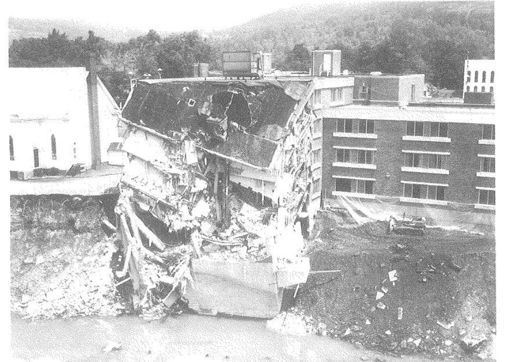
Figure 3. Damage to the Jones Memorial Hospital on N. Main St. caused by Tropical Storm Agnes, June 1972.
